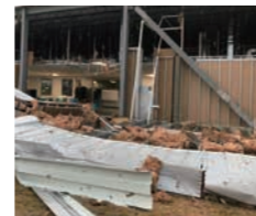
Damage caused by the tornado at the U.S. base
